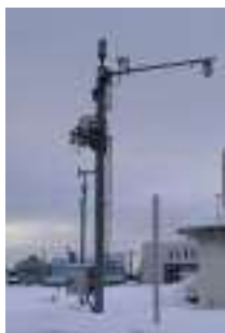
Road weather station
