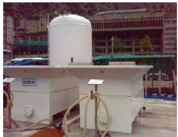
14- Brine production station
