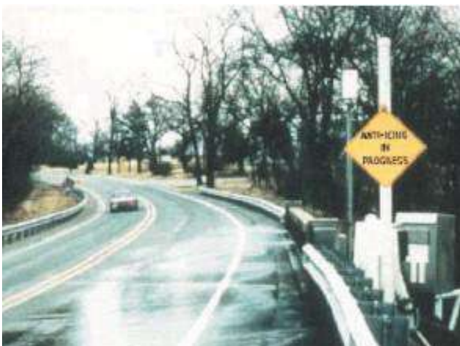
Fixed Anti-Icing Spray System (Photo courtesy of CRYOTECH Deicing)
