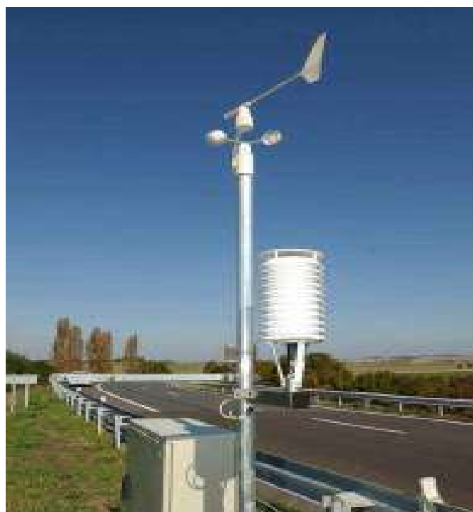
Road weather information system.
