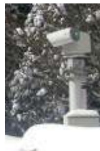
Road surveillance camera
